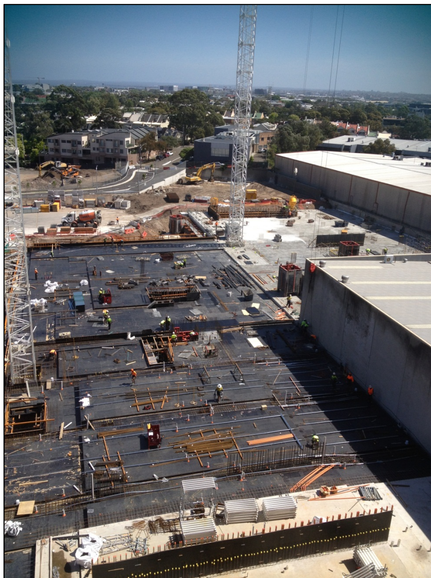
Figure 4: Construction works currently underway on site for Stage 2 (known as Buildings C and D)
